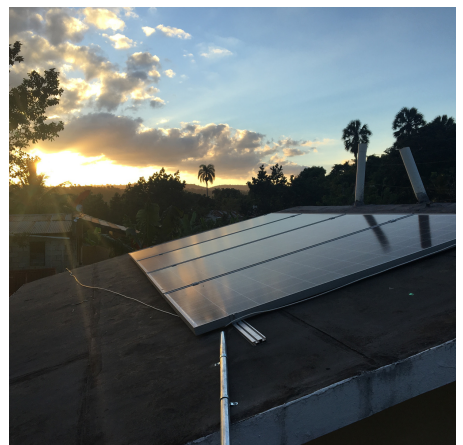
The sun shining off of the solar panels installed in December 2017 in Los Peladeros.
